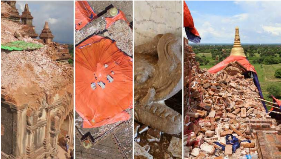
Figure 3 Examples of highly damaged heritage structures in Bagan after August 2016 earthquake.
