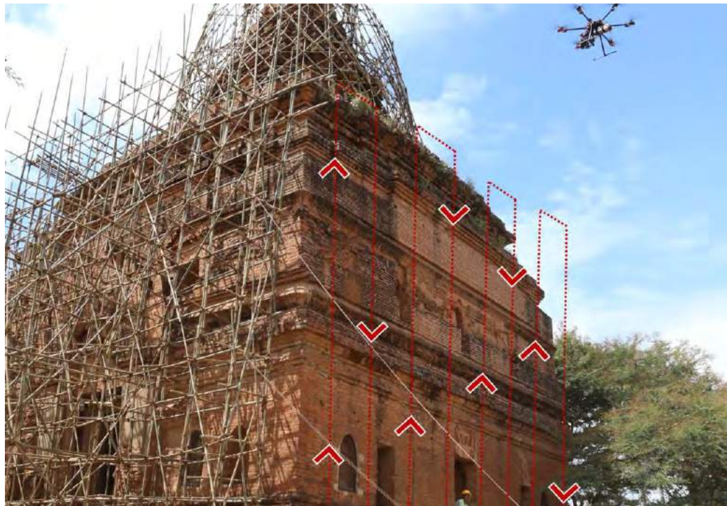
Figure 22 Example of the flight path of the drone in manual mode to capture details of the upper parts of a monument difficult to take through terrestrial photogrammetry. Image source: Author.
