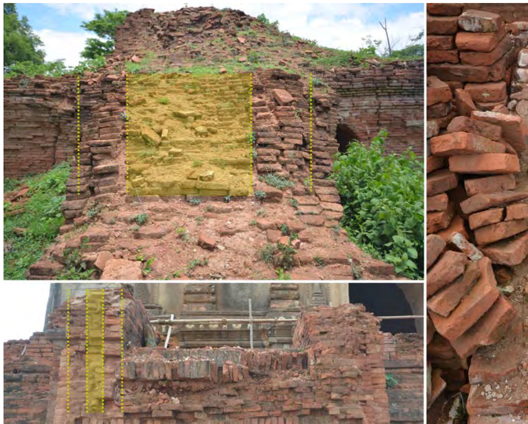
Figure 49 Visual analysis of collapsed Bagan structures. These helped to understand the employed assembly of the construction materials. Images source: Author.
